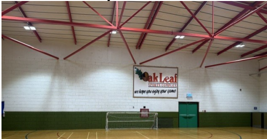
Picture 1 – Sports Hall Back Wall
