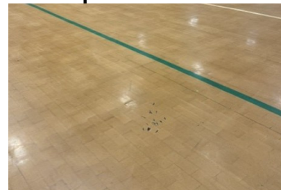
Picture 2 – Sports Hall Minor Damage
